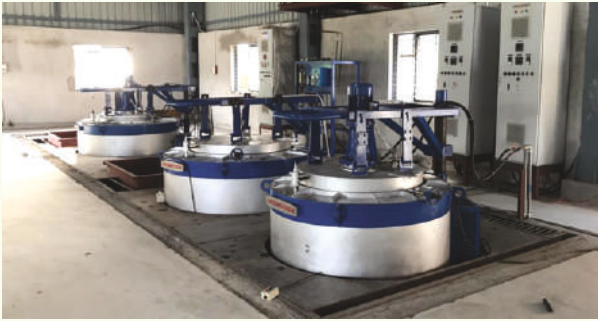
1 MT Pit Type Heat Treatment Furnace
