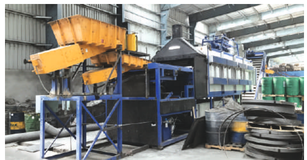
Mesh Belt Furnace
